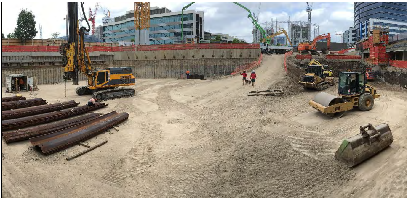
Haven Site: A ramp to the lower basement level has been established to provide access for heavy machinery.
