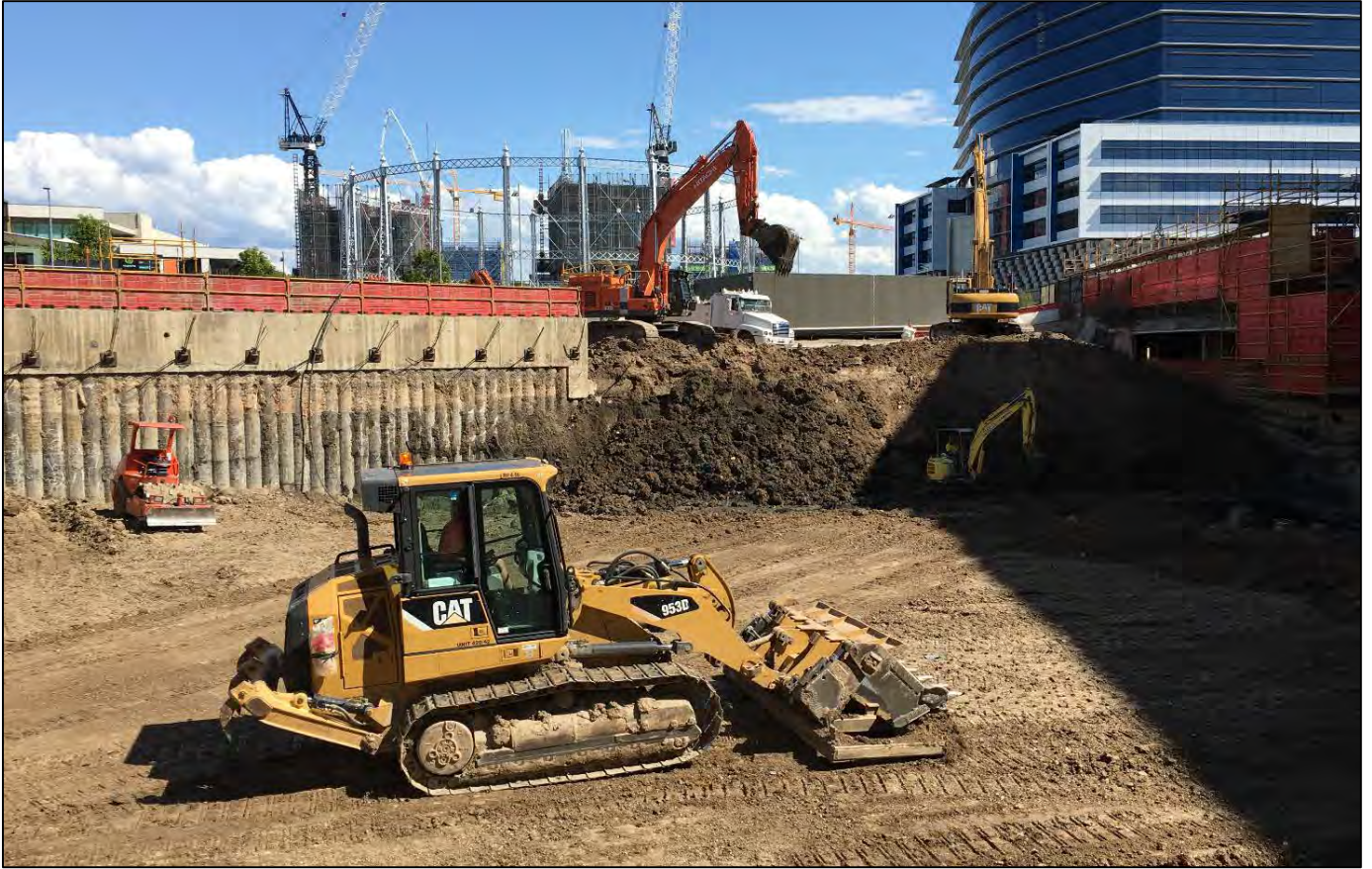
Haven Site: Remaining soil is excavated and a level platform is established for the piling rig to commence foundations.
