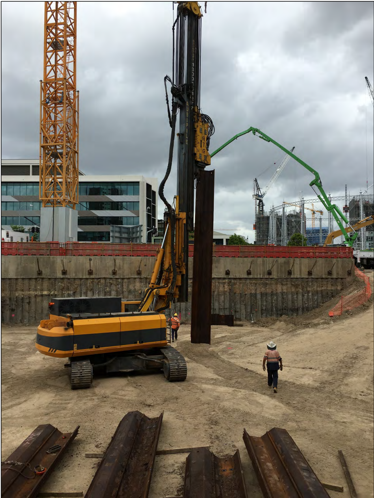
Haven Site: A piling rig is used to construct a sheet retaining wall to from the lift overrun.
