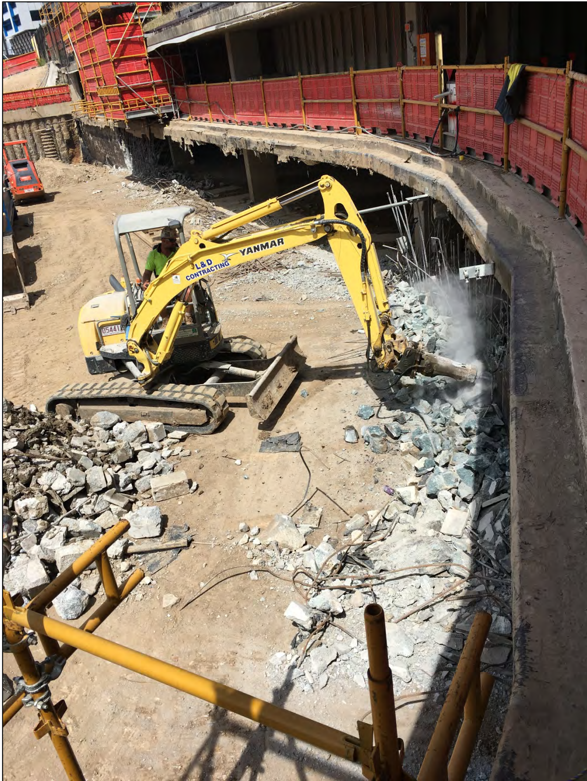
Haven Site: An excavator with jackhammer tool punches through to the pre-built car parking chamber under the adjoining Energex building.
