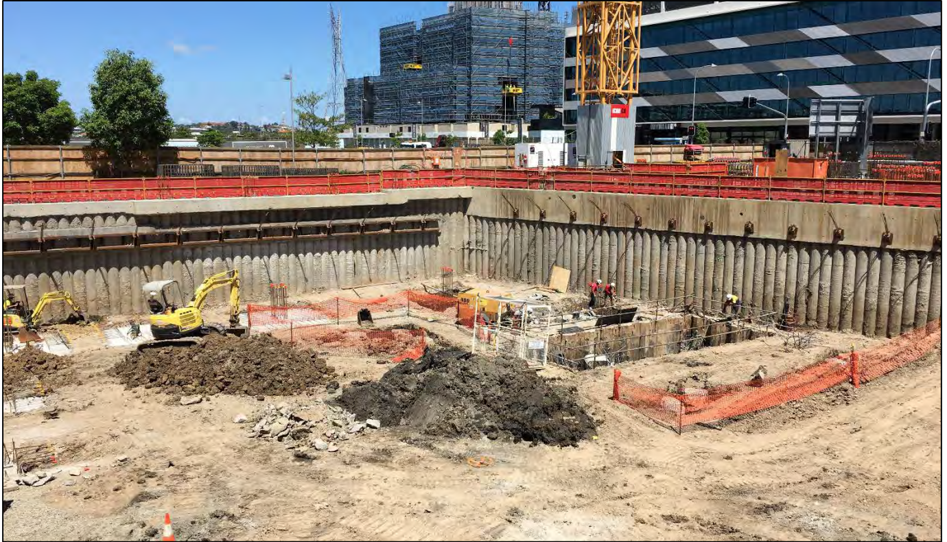
Haven Site: The hole is retained for the base of the lift well which will continue, non-stop to the 25 th level roof terrace.
