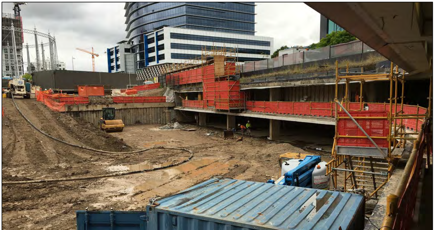
Haven Site: Construction continues in muddy conditions. The basement 2 chamber is now fully accessible. The red fencing screens form part of the worker access ramps to the site offices.
