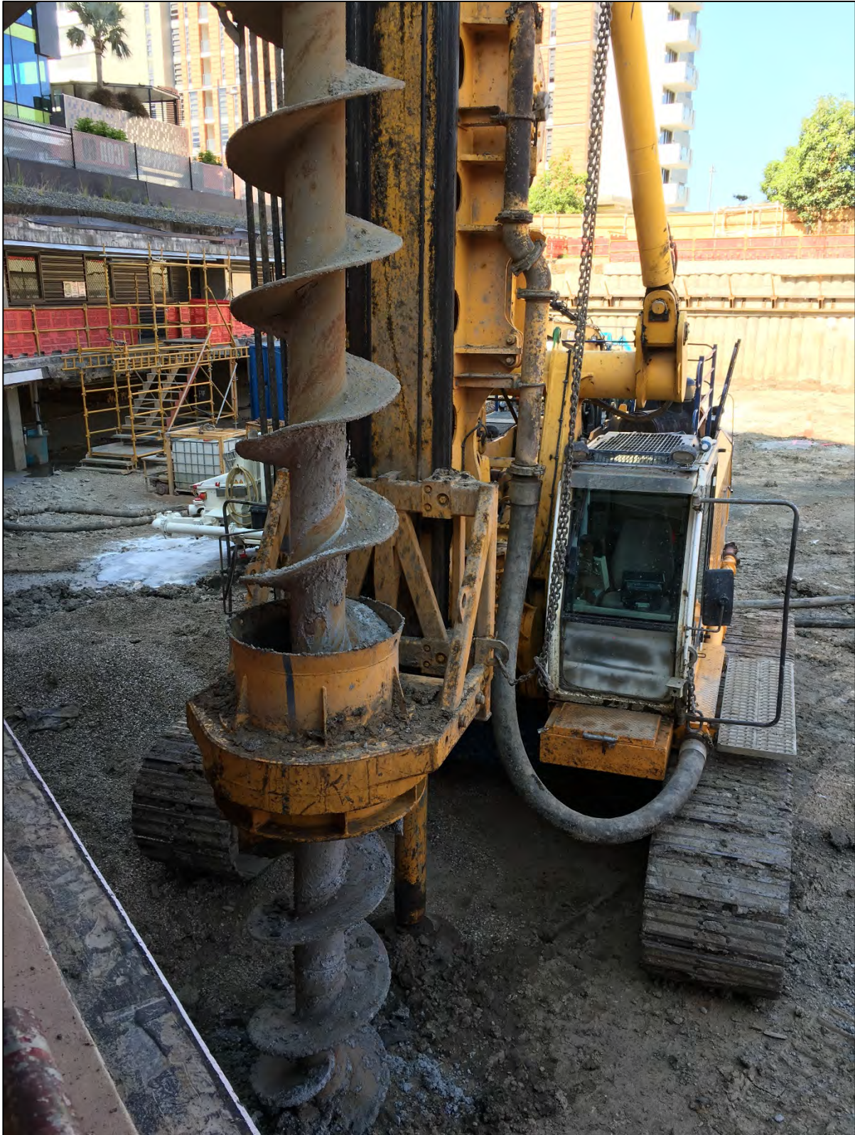
Haven Site: One of the piling machines used to construct the basement foundation piles.
