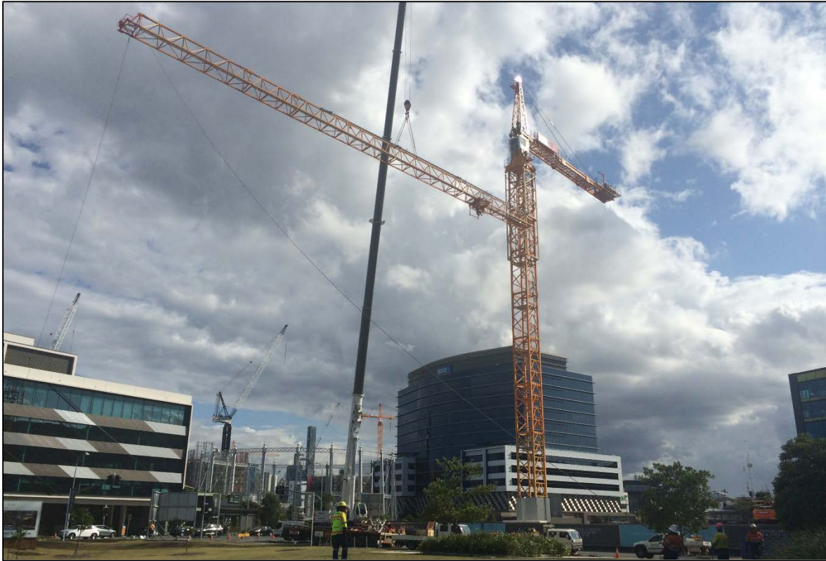
Haven Site: The tower crane was delivered to site in several pieces and erect over the course of a weekend.
