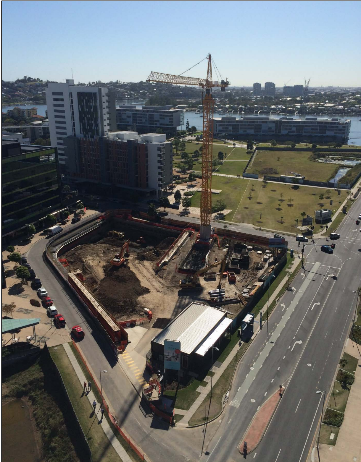
Haven Site: The development team are installing cameras to provide live photography of the construction process. Access will be available via the Haven website in the coming weeks.
