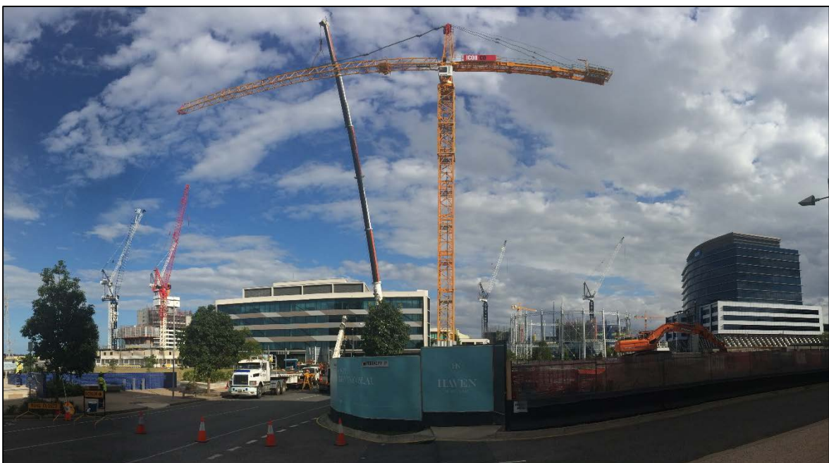
Haven Site: Icon's tower crane is commonly referred to as a 'hammerhead crane' which includes a fixed jib (crane arm). Nearby developments are utilizing 'luffing cranes' that can navigate over nearby obstructions and adjoining developments.
