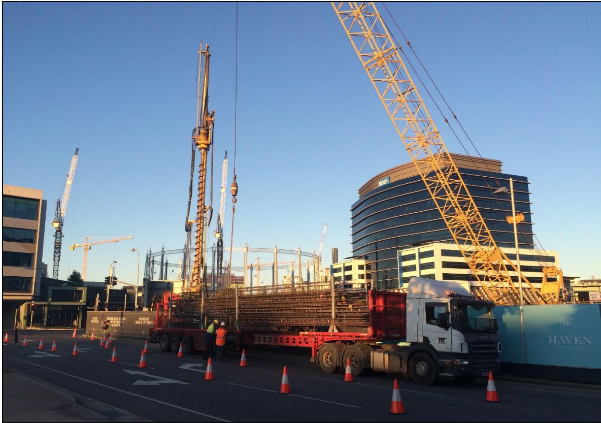
Cunningham Street: Traffic control in place while crane lifts steel reinforcing over hoarding onto site for use in pile foundations.
