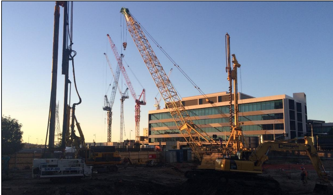
Haven Site (left to right): Concrete pump, piling rig, crane, 30 ton excavator, drill rig.
