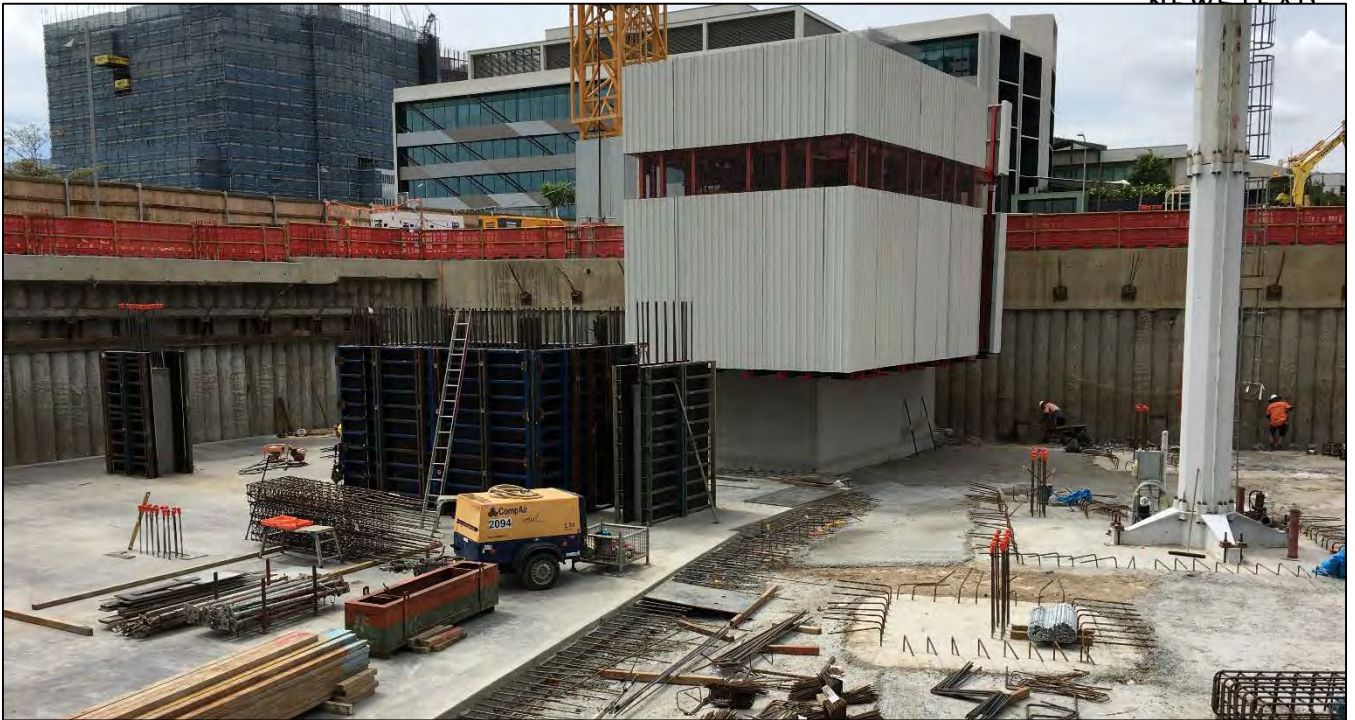
Haven Site: The jump form system is established around the lift well and formwork is prepared for the basement column supports.
