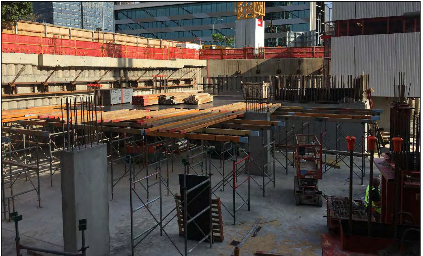
Haven Site: Formwork is prepared for the Basement 1 slab pour scheduled for January 2016.
