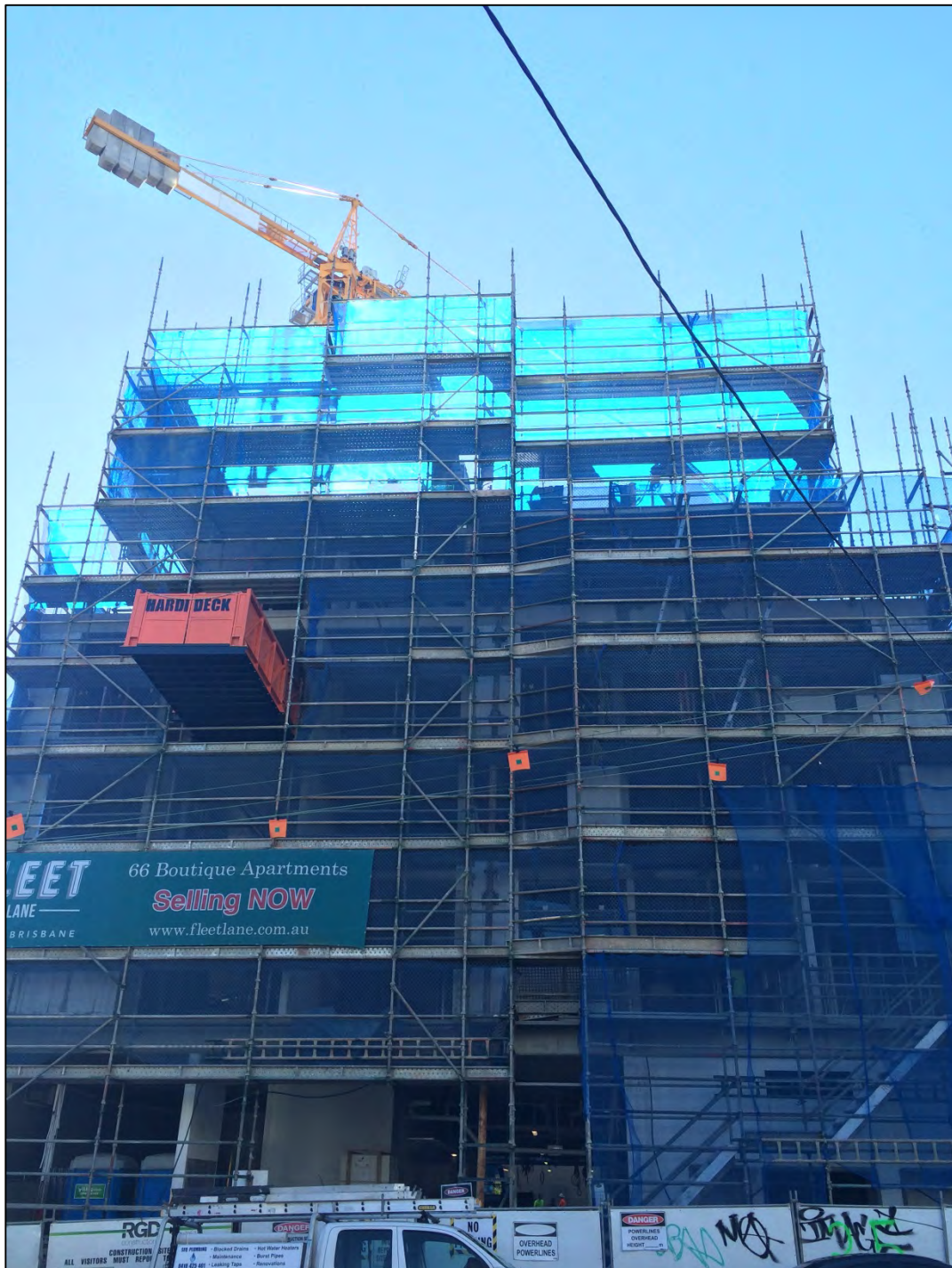
Figure 2: View from the Hope Street Frontage. Construction has progressed beyond the podium levels and now continues on the tower component. Progress is expected to accelerate with this phase now underway.
