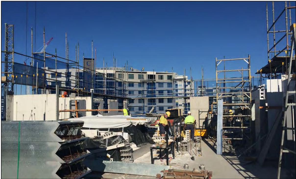
Figure 4: Roof Top – Erection of structural walling. Building materials for all walls, including non-structural walls, are stored on each level while access is available. The non-structural walls will be erected while construction continues above.
