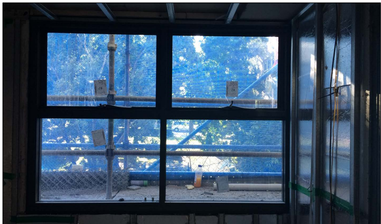
Figure 9: Level 2 – the first glazing panel inserted at Fleet Lane. In future, this will become the park view from the master bedrooms.
