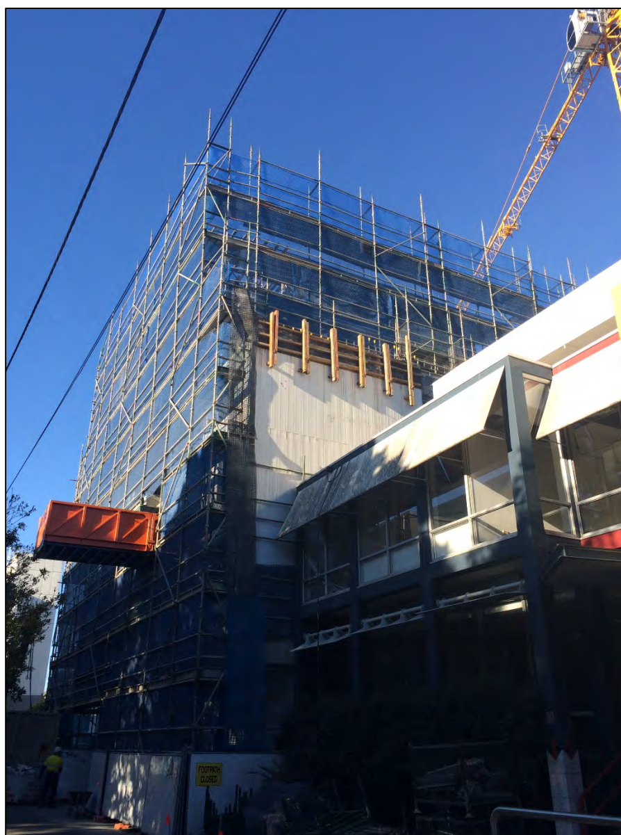
Figure 1: Site as viewed from Fleet Lane. The orange projection is a material loading bay used for loading building material to areas were required. It is an efficient way of transporting materials to where they are needed.
