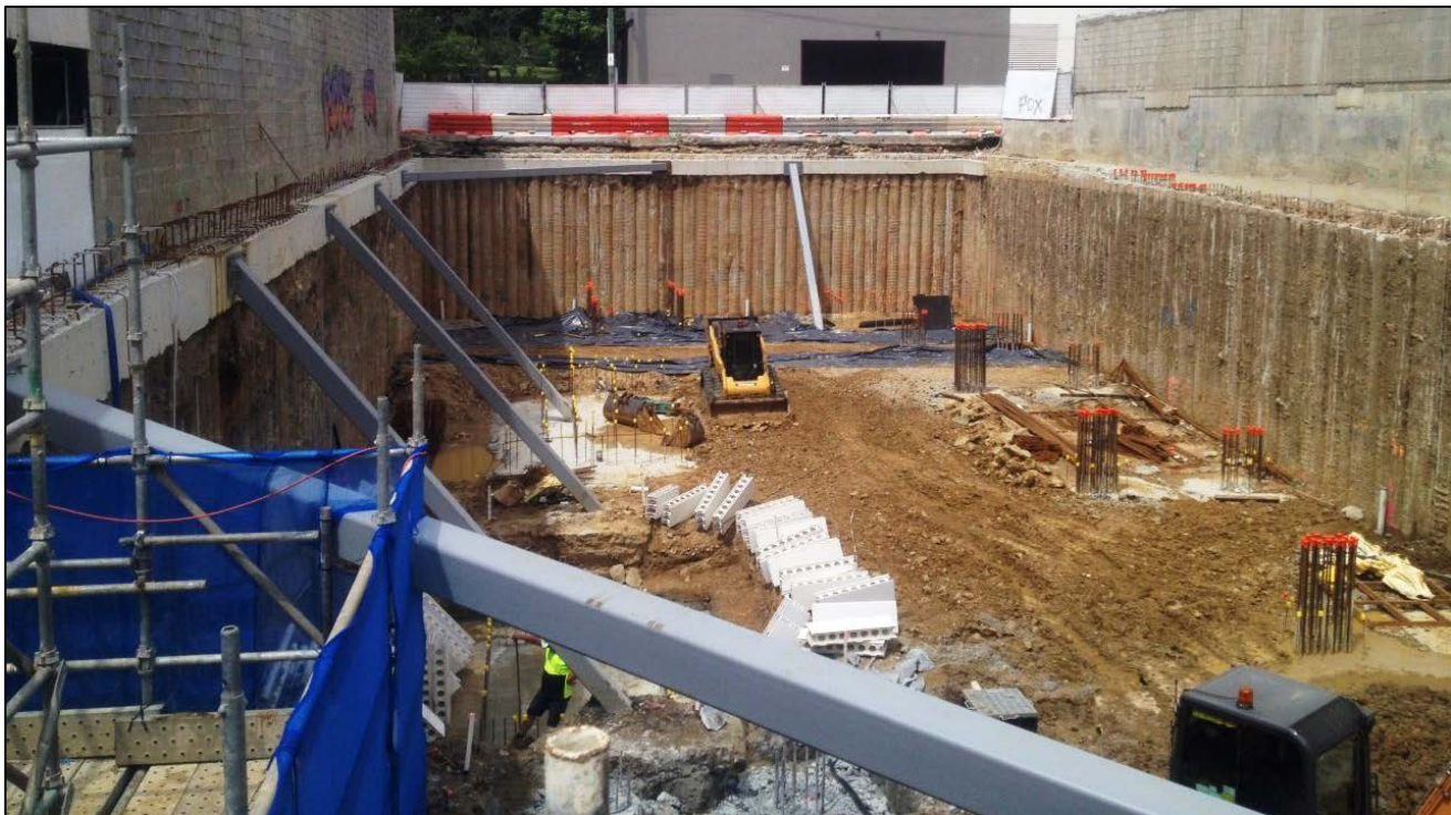
Figure 4: Following excavation of the site, the foundations are poured in preparation for the basement 2 slab.
