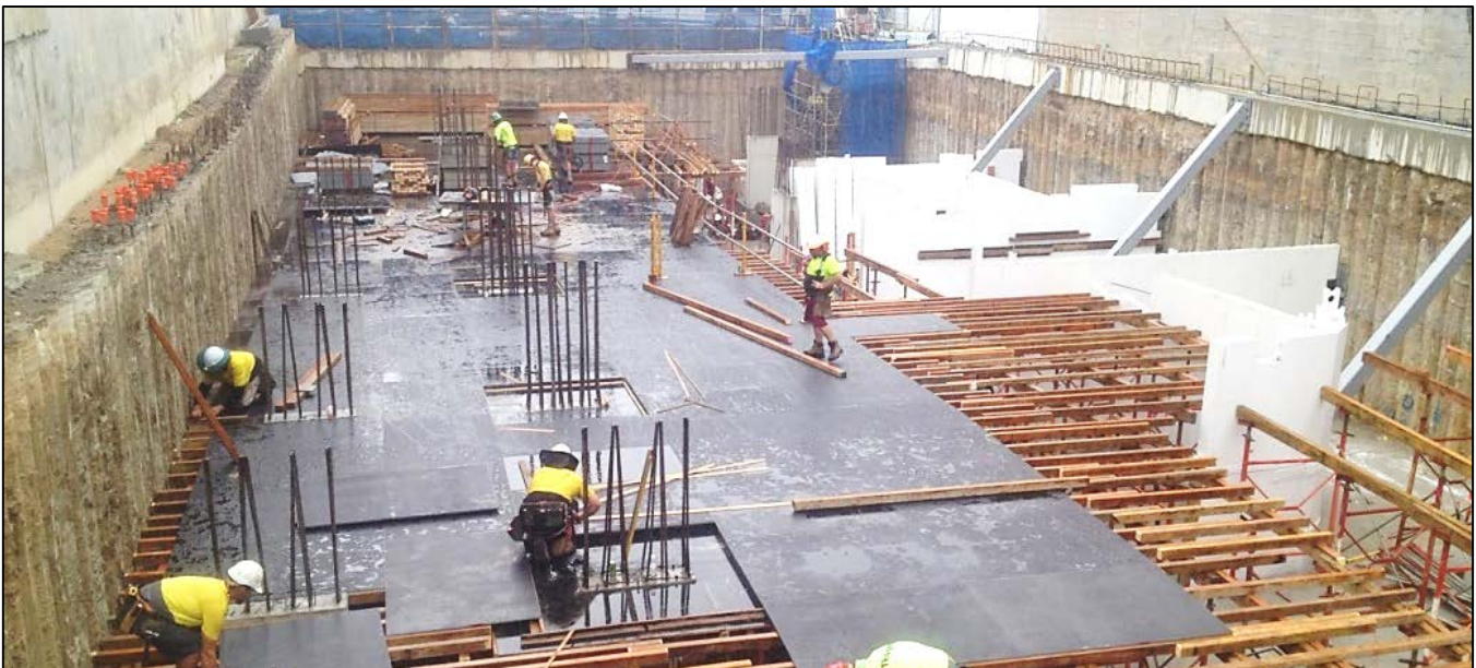
Figure 6: Once the basement 2 walling system is erected, the formwork is prepared for the basement 1 slab.
