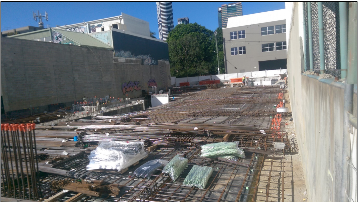
Figure 8: Reinforcing mesh was prepared this week in preparation for the ground floor slab pour, a major milestone in the construction timeline. The risk of delays in the construction period are largely reduced following the ground floor slab pour.
