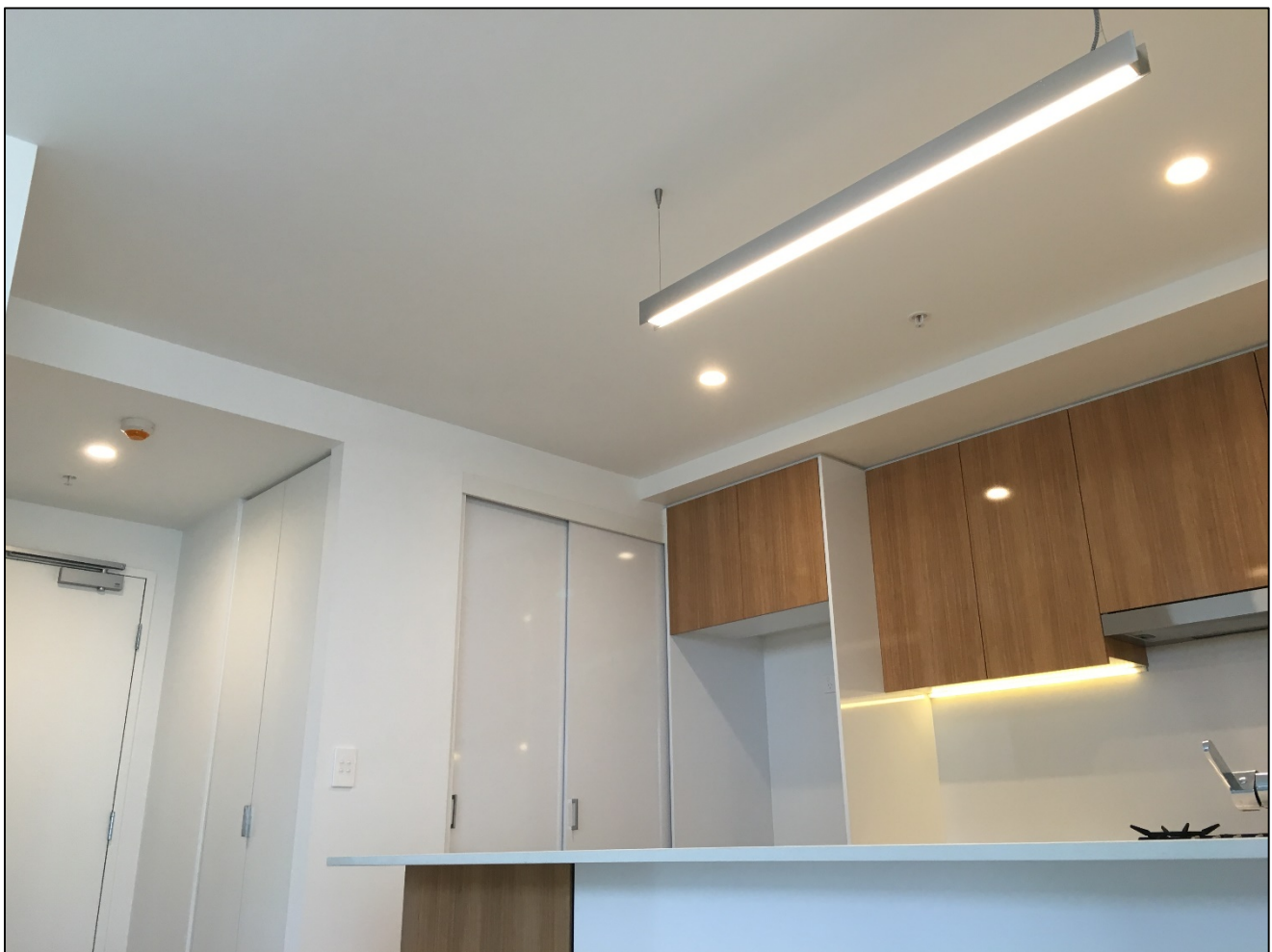
Figure 2: Fleet Lane Typical Apartment Lighting – Recessed LED Down Lights.
