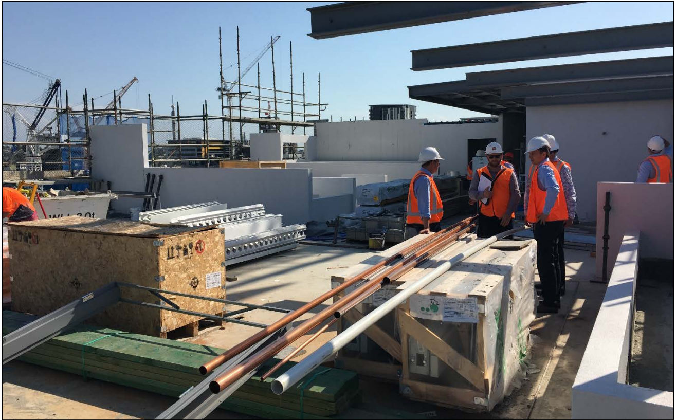
Figure 2: Fleet Lane Rooftop – Inspection of the roof top by the super intendent, architect, project advisors and quantity surveyor.
