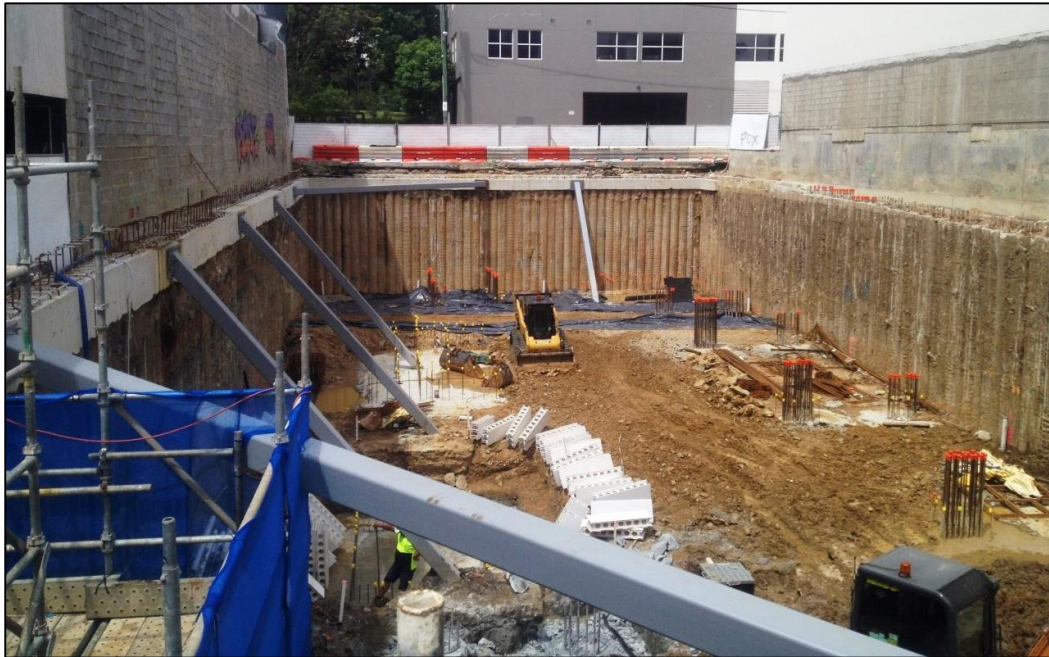
Figure 2: The black plastic sheeting on the Fleet Lane frontage is lining a temporary pit designed to capture and drain any rain water. The water is pumped out and the site is primarily kept dry allowing construction to progress.
