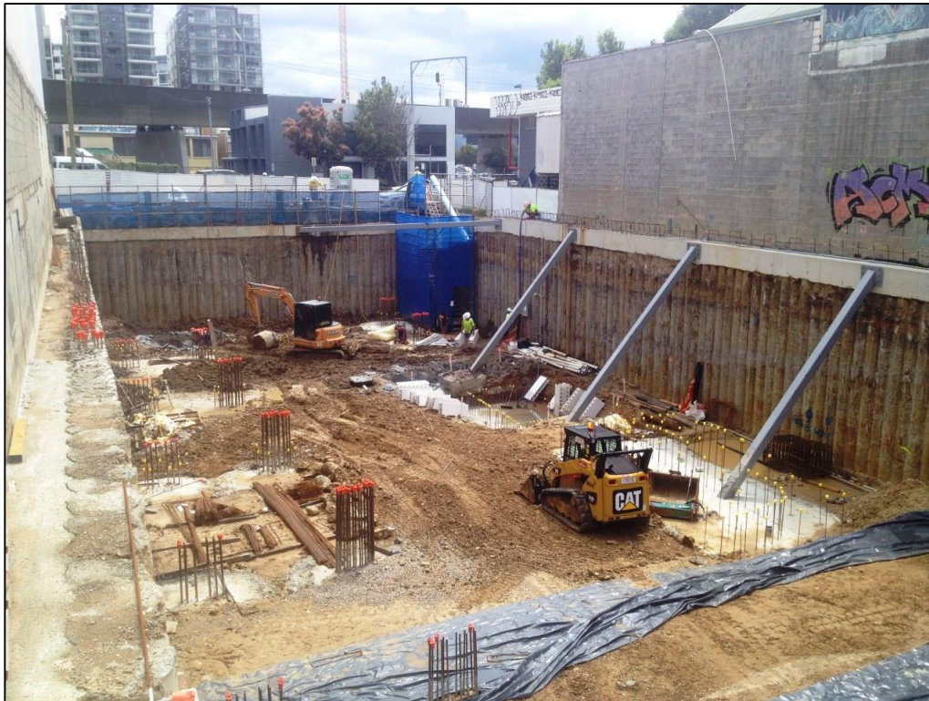
Figure 1: Despite recent rain events, all soil has been removed from site. Steel bracing has been installed to stabilize the retaining wall while the basement levels are under construction.
