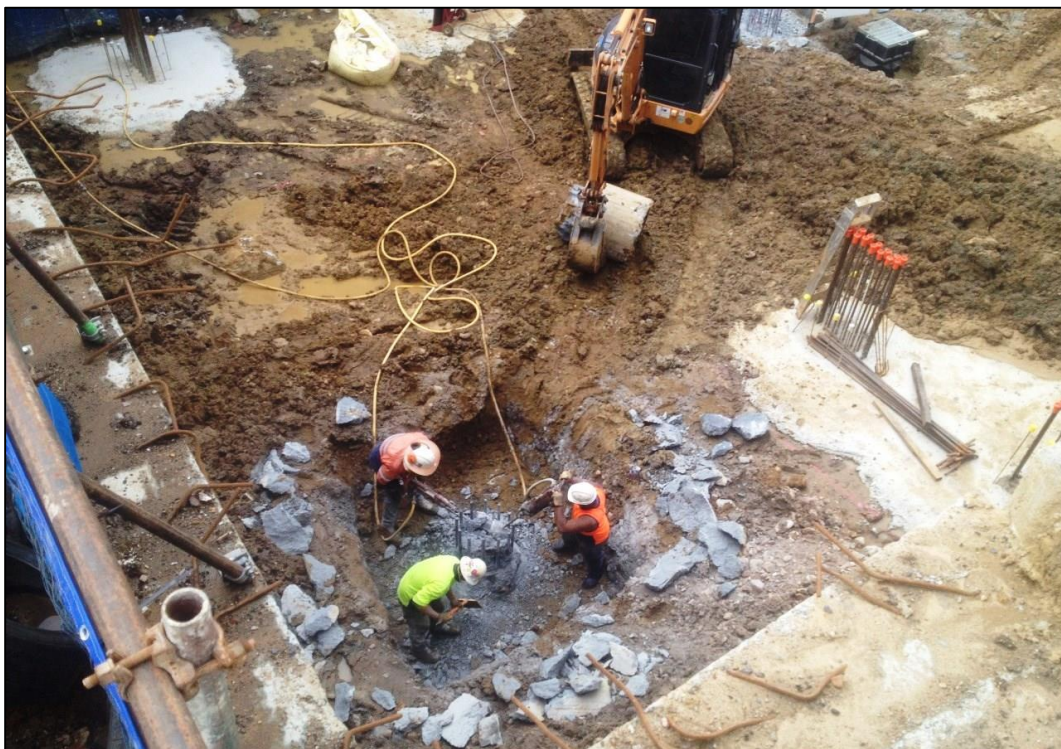
Figure 3: The top of the pile is removed to expose the steel reinforcing which is then integrated into the pile cap. Once inground plumbing is complete, the Basement 2 floor slab is poured.
