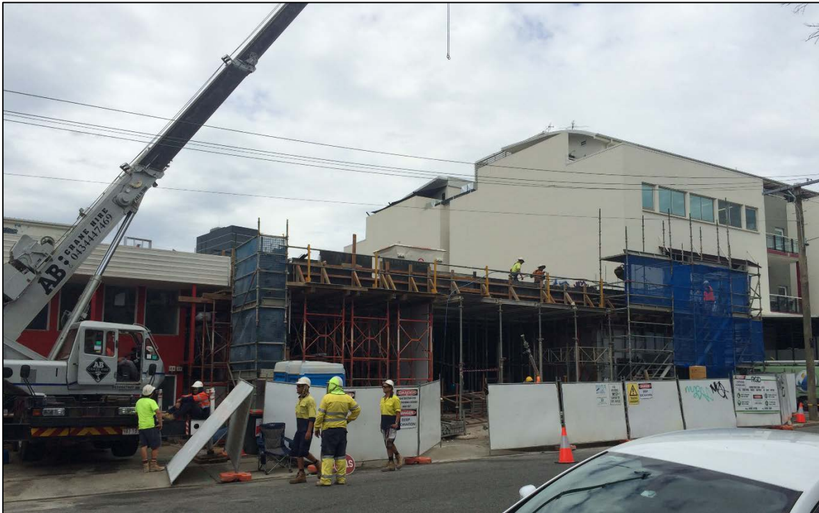
Figure 1: Site as viewed from Hope Street. Scaffolding and formwork inplace for the level 2 slab pour. Level 1 shows the beginnings of the lobby entrance to the left, and the café style tenancy in centre.
