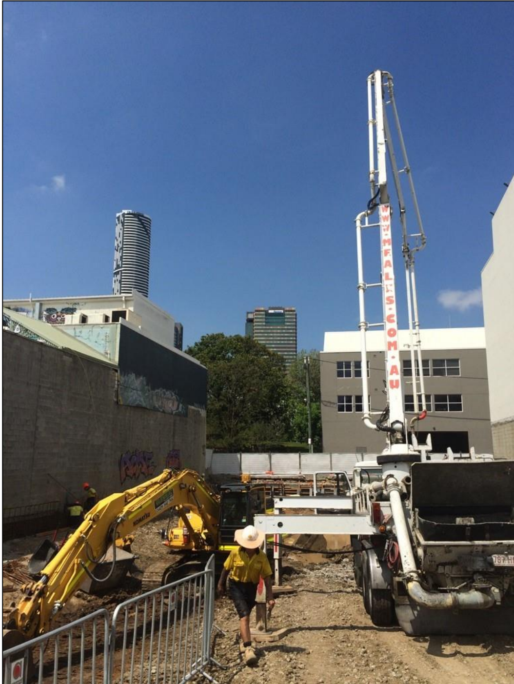
Figure 4: A concrete pump extending to the Fleet Lane frontage to pump concrete to form the capping beam.
