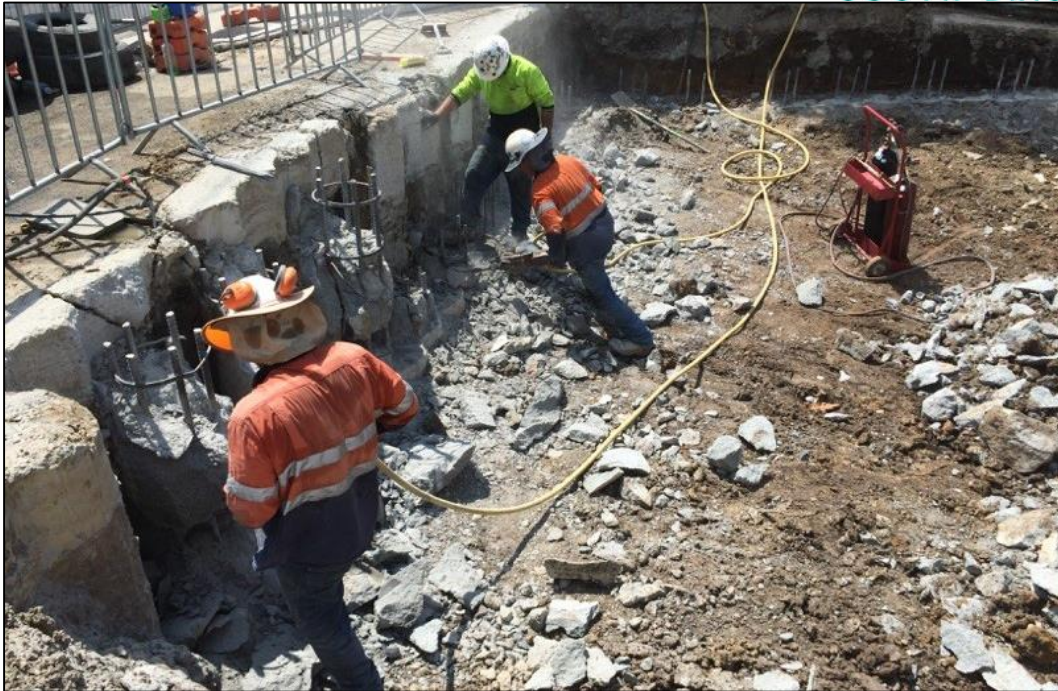
Figure 2: The secant retaining wall system consists of a continuous concrete pile system. Workers are removing the tops of the piles, exposing the steel reinforcing so as to pour a capping beam to connect and strengthen the retaining system. Once this is complete, excavation for basement levels can begin.
