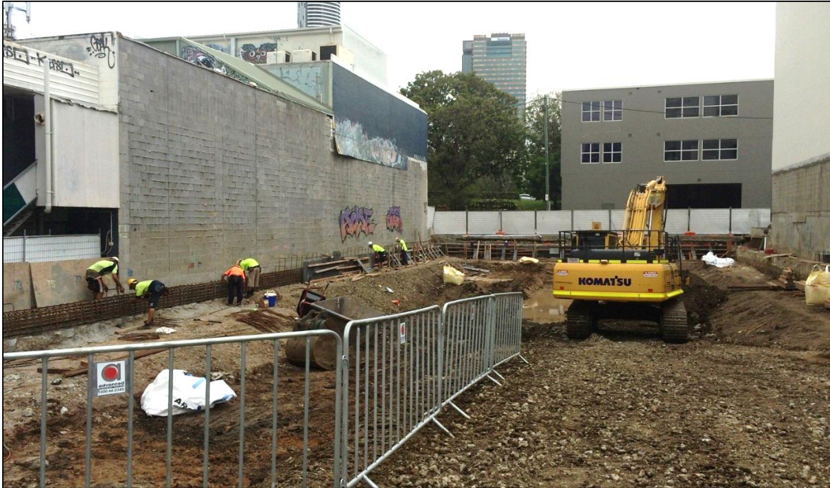
Figure 1: Despite recent thunderstorms, the site works are progressing well. Water in the background is the result of recent storms and site water is intentionally collected in an area of the site not currently under construction. It will be pumped to water trucks and disposed from site.
