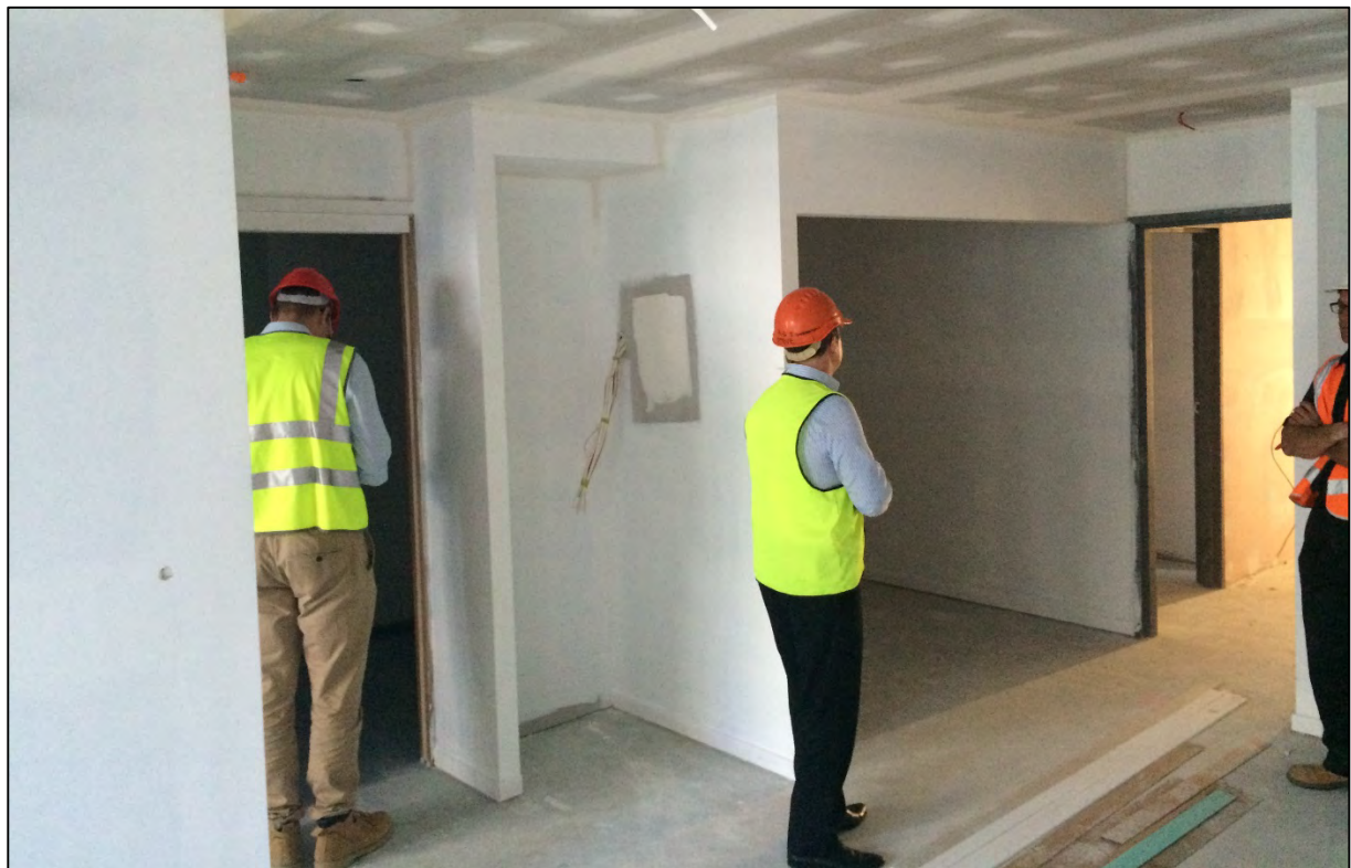
Figure 3: Inspection of proposed prototype apartment on level 2. The first coat of paint has been applied to walls.
