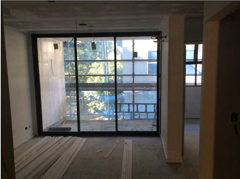
Figure 4: Level 3 is now completely sealed with all windows and doors now installed.
