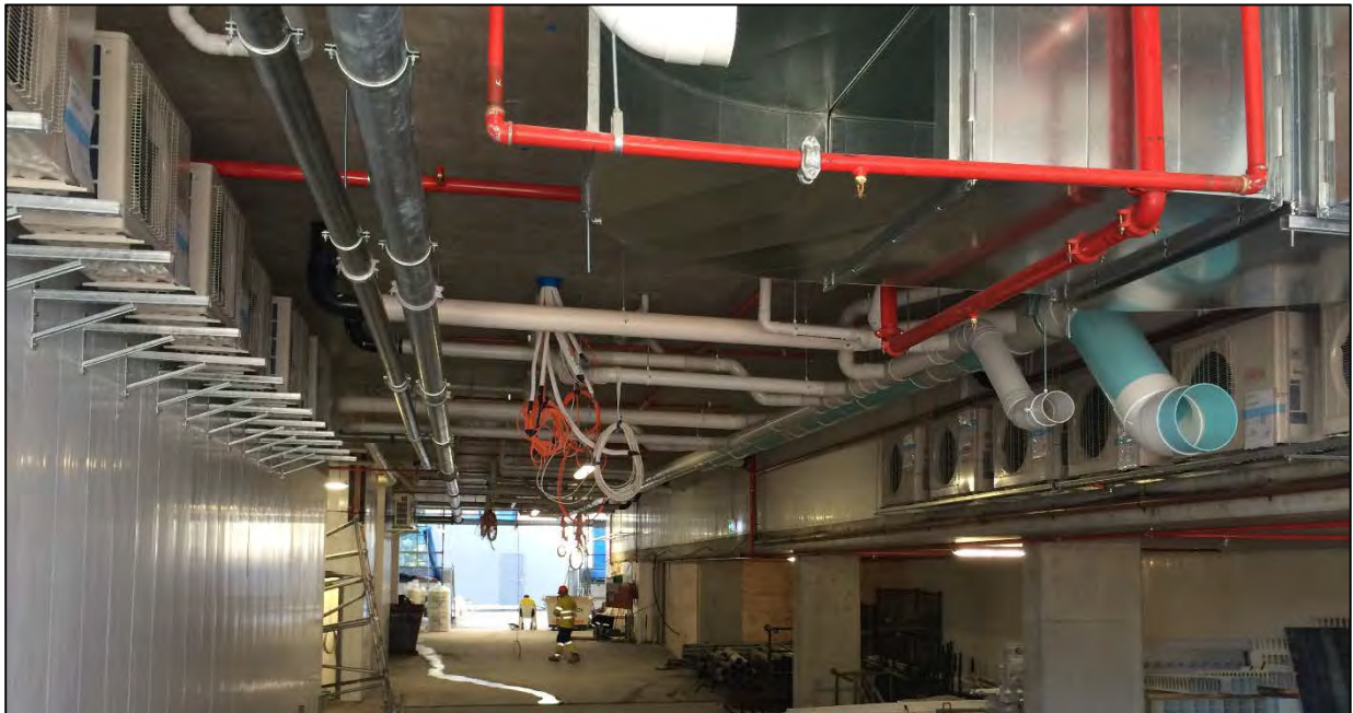
Figure 2: Ground floor driveway from Hope Street frontage showing the recently installed air condensers to supply air conditioning to the podium levels.
