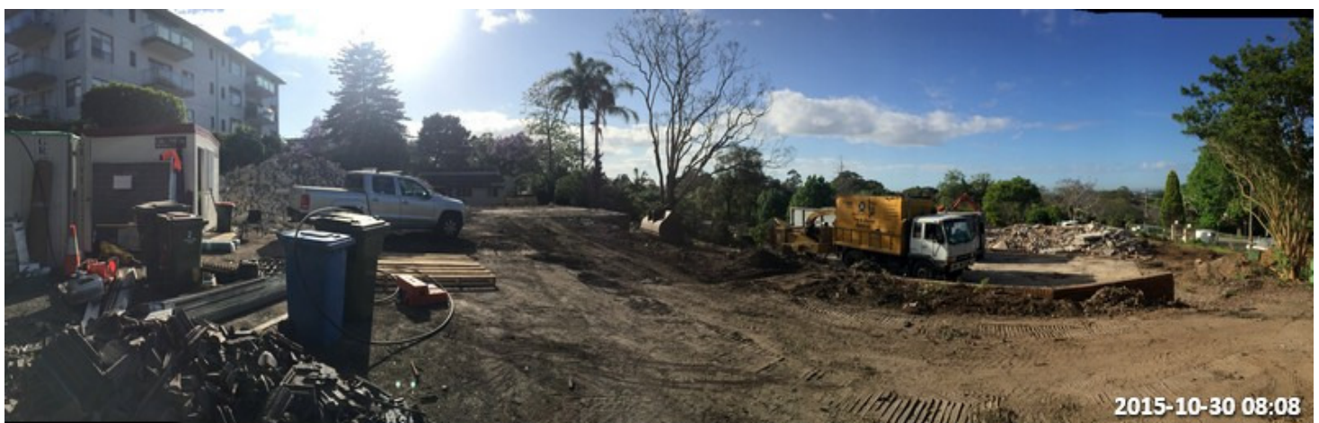
Photo 6 – The photo below shows panoramic view of the demolition progress of the upper level section of the site from 2 Livingstone Avenue. The Builder has completed demolition of Livingstone Avenue properties and now focusing on 1 Orinoco St and 1074 Pacific Highway Properties with target completion within 2 weeks.
