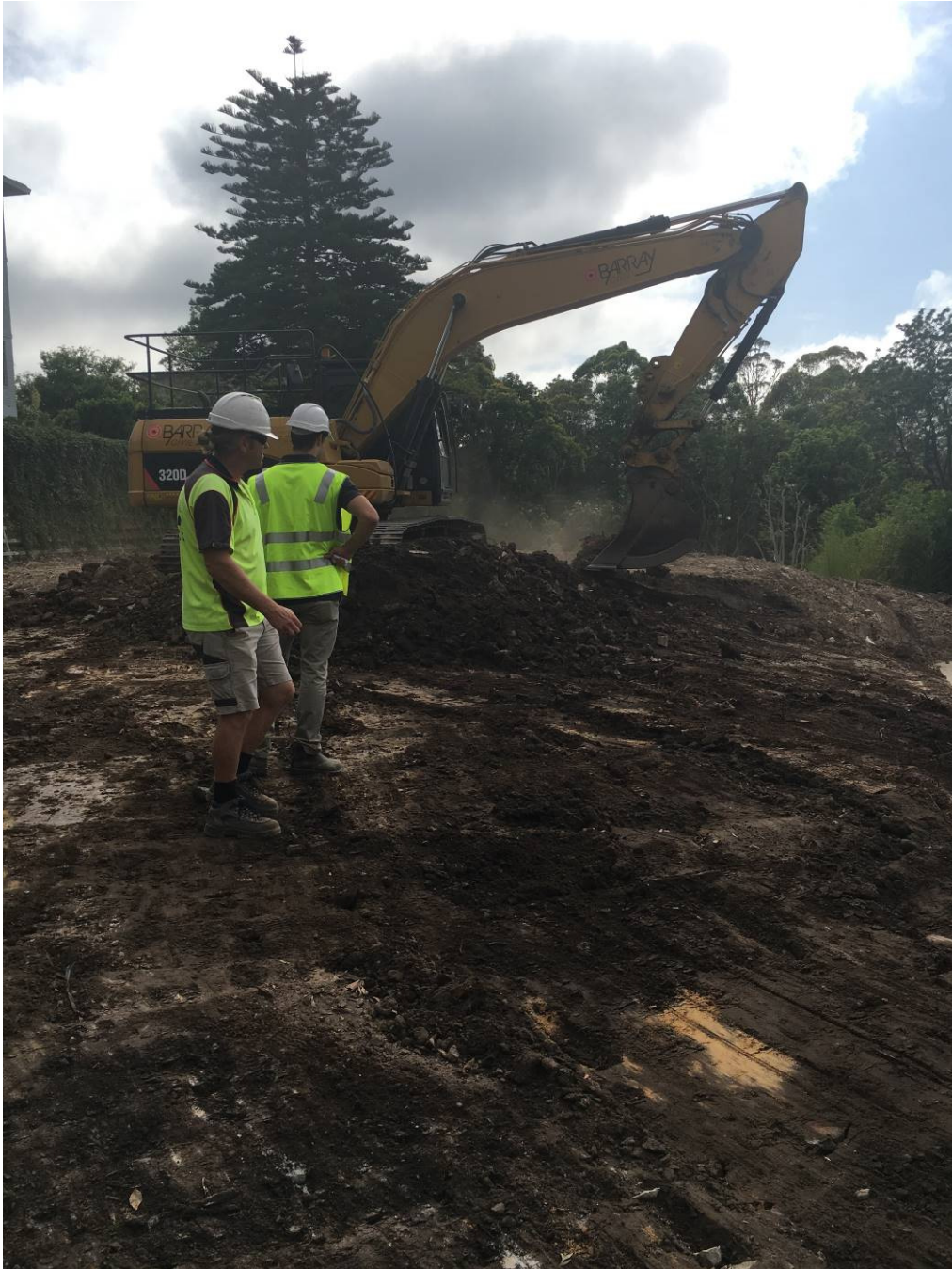
Photo 3 – The photo below excavators stripping off the top fill layer for screening and disposal.
