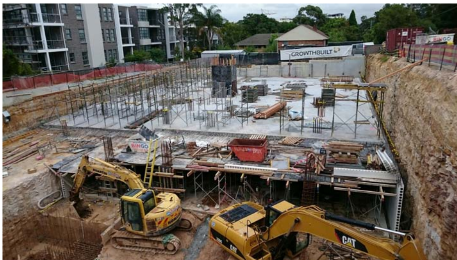
Photo 5: The Ground Floor western side's suspended slabs frames and bearers formwork have been installed.
