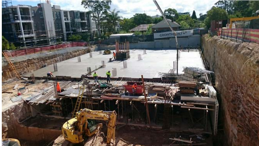
Photo 4: Completion of the concrete pour to the Basement One west side suspended slab.
