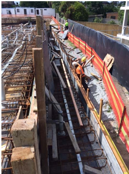
Photo 6: The below shows the deep rebate in the slab to the rear of the project. This set down is the location of the deep soil planting to the rear of the project.
