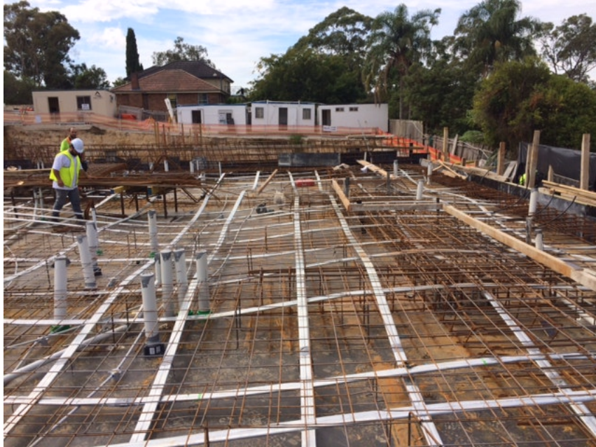
Photo 3: The ground floor western suspended slab is complete and ready for the concrete placement.
