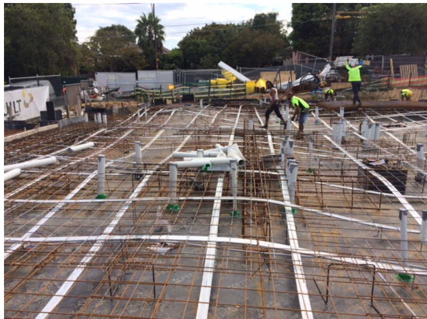
Photo 4: The last of the reinforcement mesh is being installed and fixed off. All plumbing rough-in is complete.
