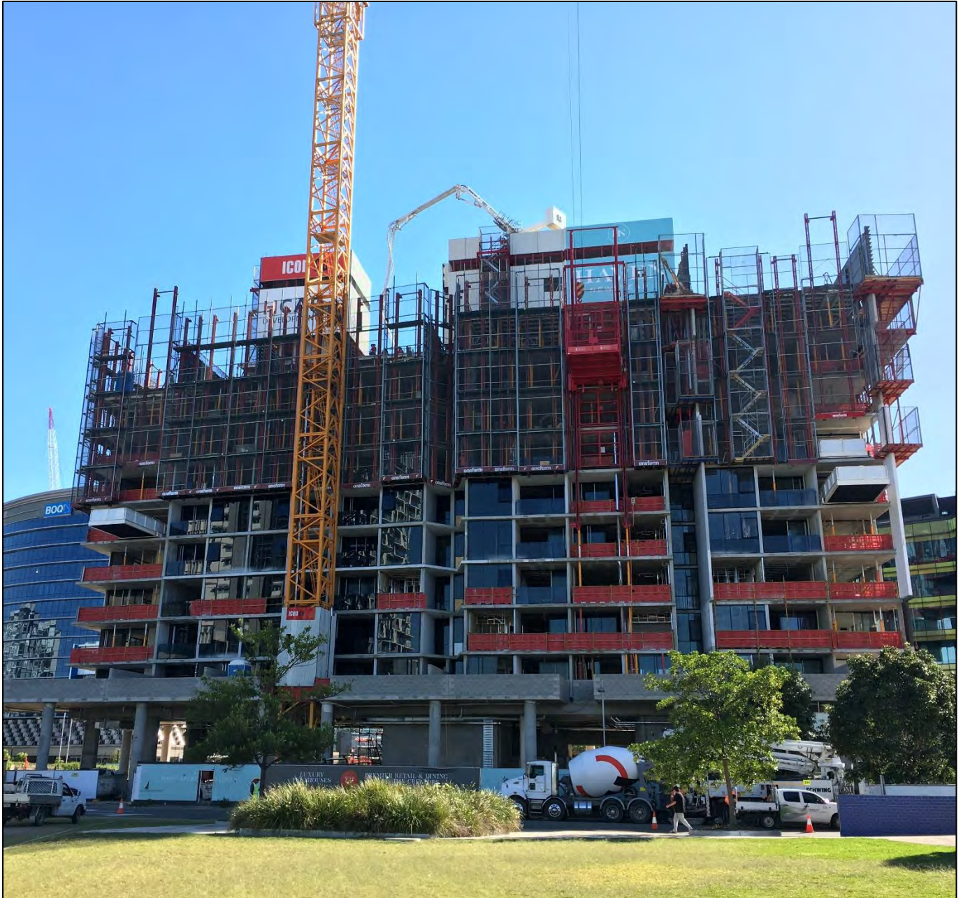
Haven Site: Eastern Elevation from Waterfront Park – Concrete is pumped from trucks on Cunningham Street, through the building to the top Level to form structural walls.
