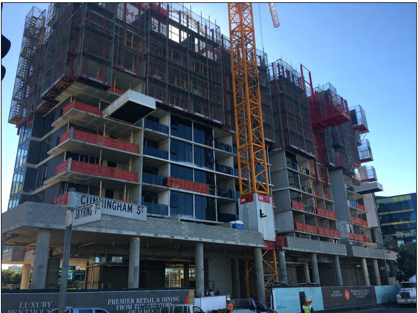
Haven Site: Eastern Elevation from the corner of Skyring Terrace and Cunningham Street.
