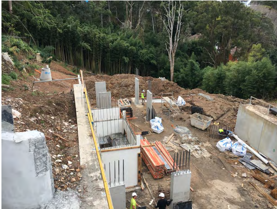
Photo 2 – The picture below taken on the 1 st of August shows building A’s foundation footings and commencement of internal walls for the fire stairs.
