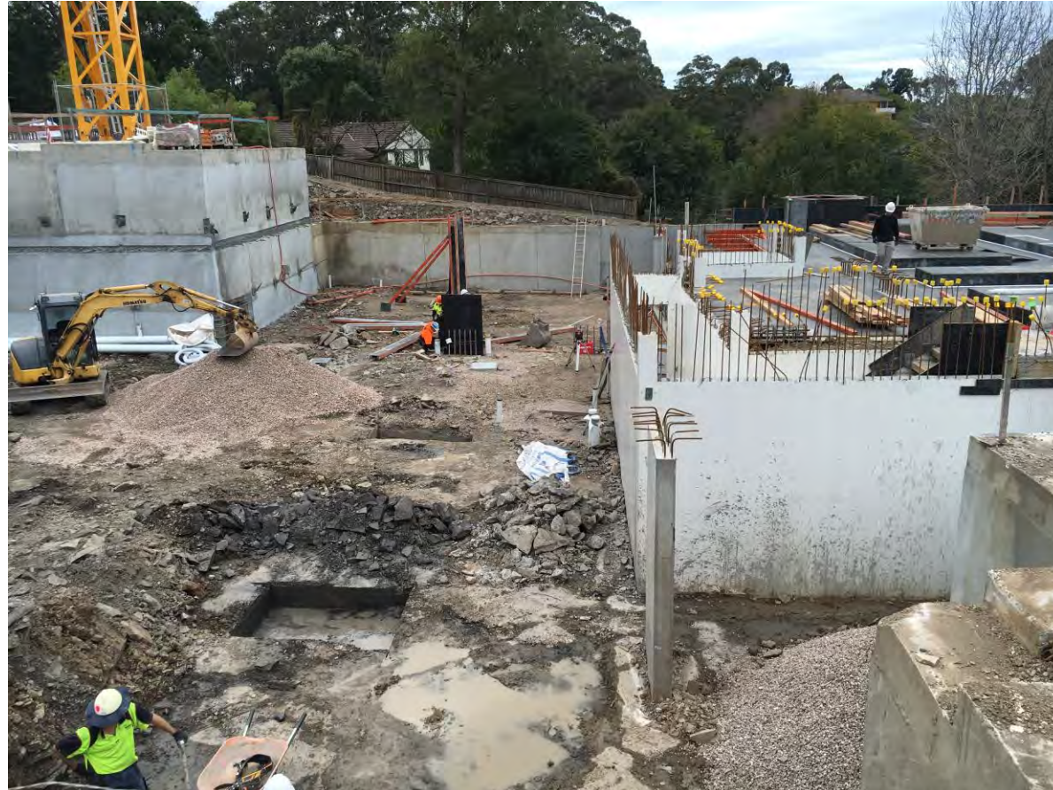
Photo 3 – The picture below from the 1 st of August show building C's internal structural walls commencing and formwork for L2 Slab.
