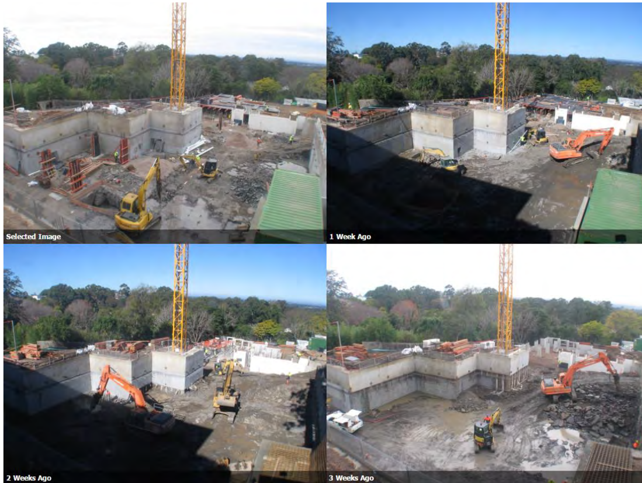
Photo 4 – The time lapse photos below show the progress of works over the past 3 weeks
