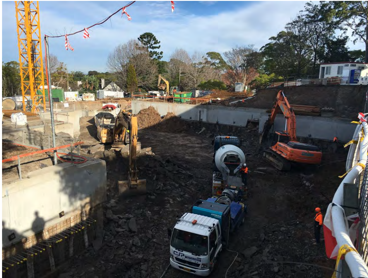
Photo 4 – The photo below from the 23 rd of June shows the extent of excavation on Building B, approximately 2-3m above the final reduced level.
