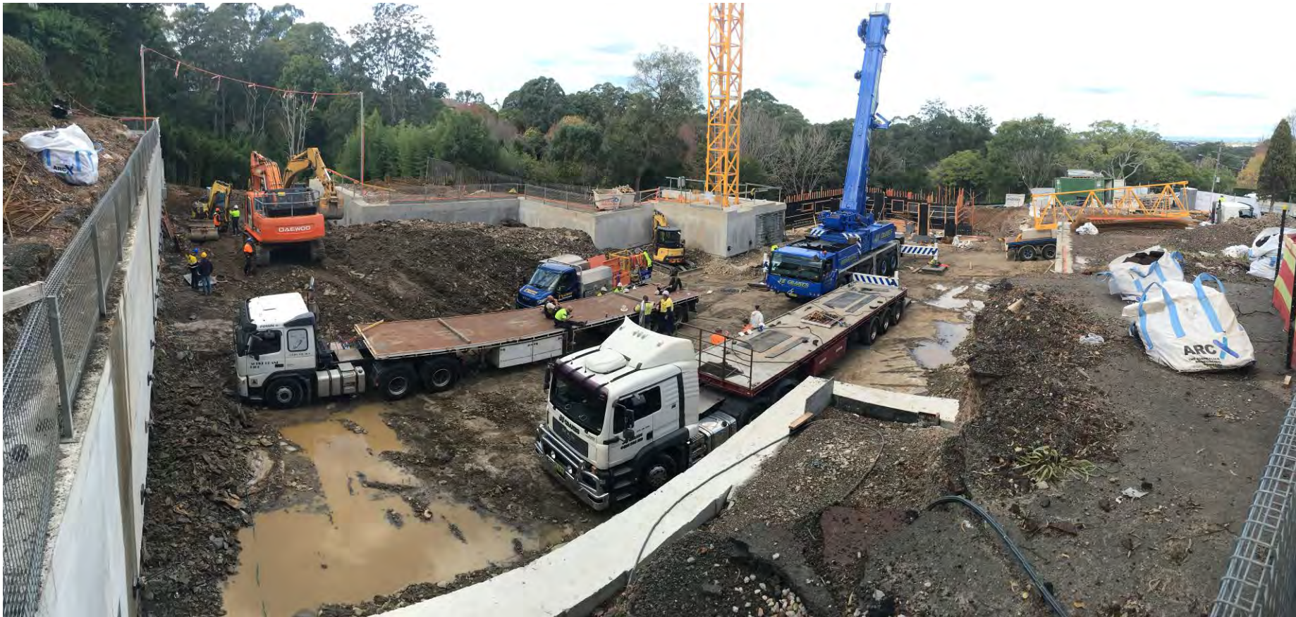
Photo 2 – The panorama below taken on the 7 th of June show the two flatbeds delivering components for the tower crane installation as well as excavation continuing in the North-East corner of the site.
