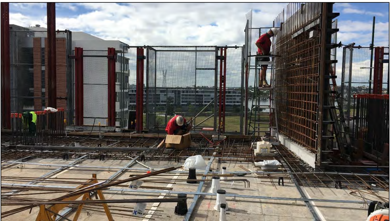
Haven Site: Easterly view to Waterfront Park from the Level 5 slab. Reinforcing and services are currently being laid.
