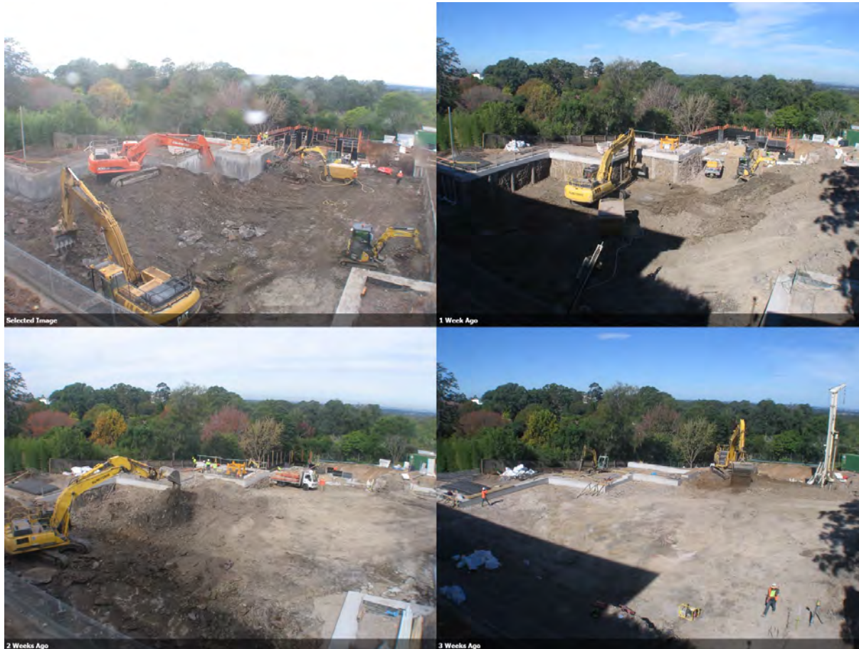
Photo 6 – The time lapse photos below show the progress of works over the past 3 weeks.
