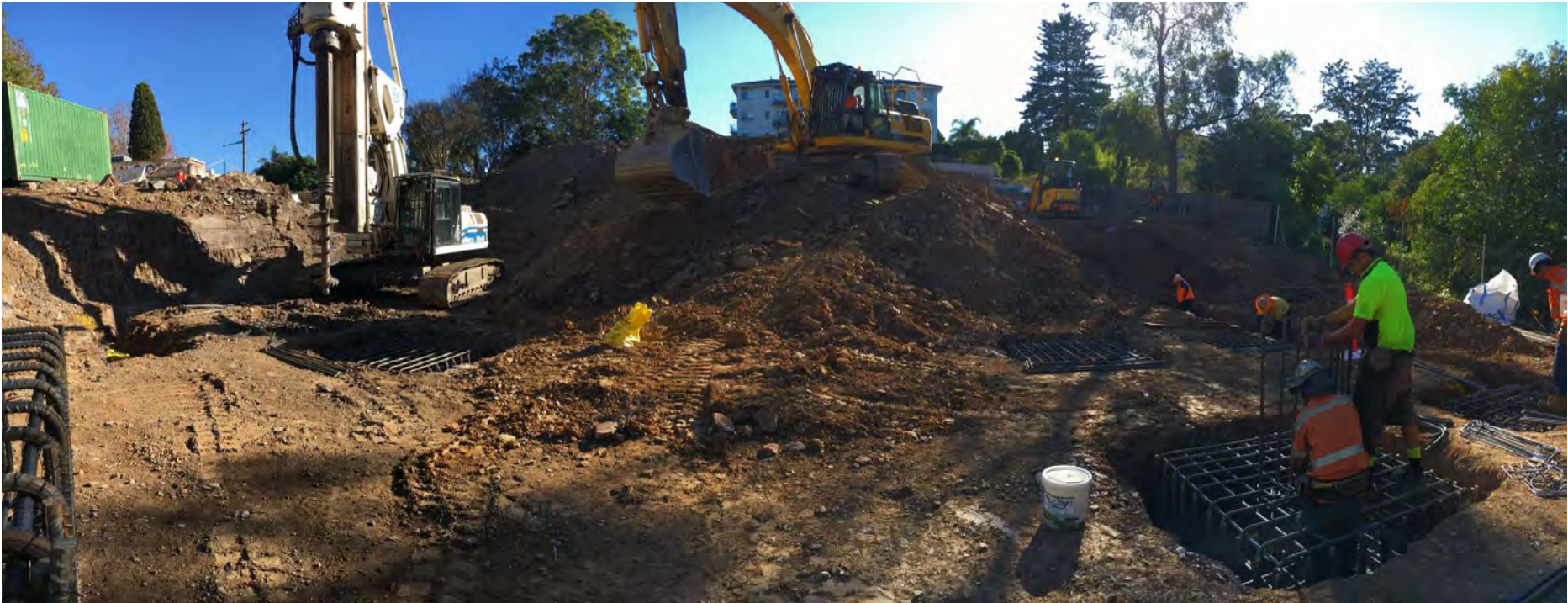
Photo 3 – The panorama below taken on the 10 th of May show the Southern corner of the sites pad footings being installed.
