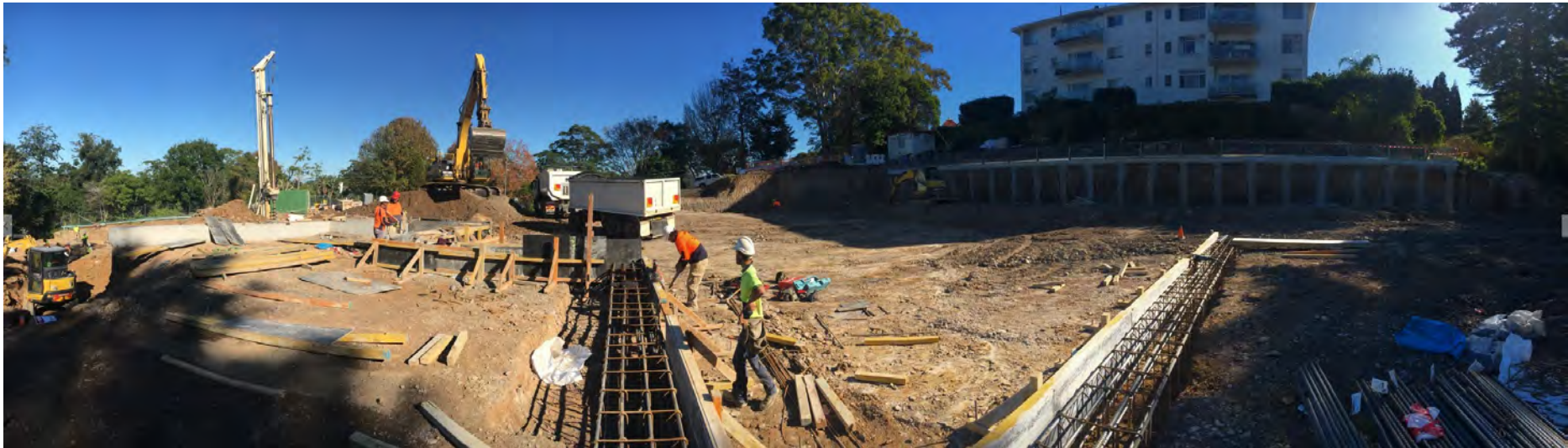
Photo 4 – The panorama below from the 10 th of May shows capping being formed in the Eastern area of the site.
