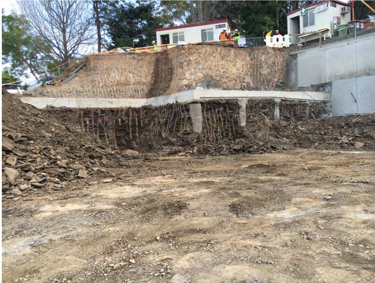
Photo 5 – The photo below from the 31 st of May shows excavation in the North West corner of the site.
