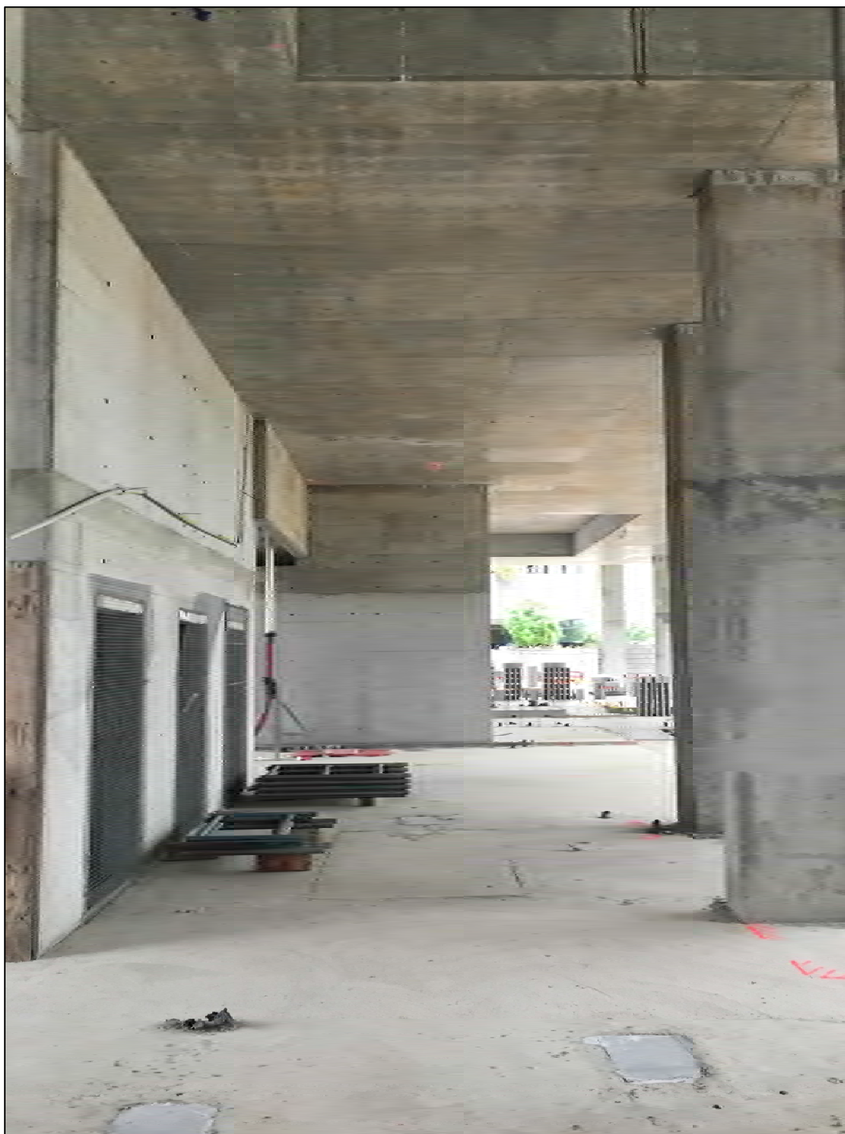
Haven Site: With back-propping now removed, the resident lobby area is revealed.
