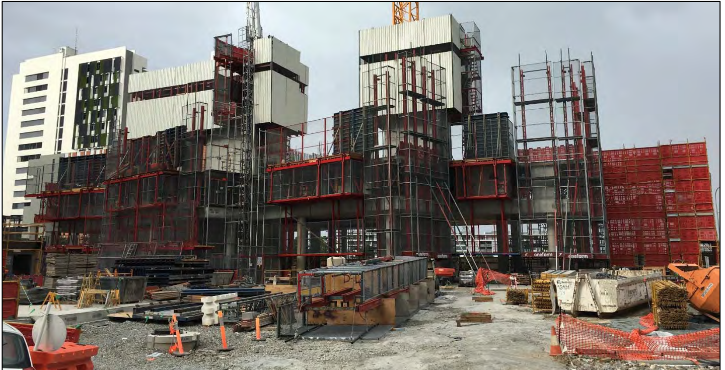
Haven Site: Easterly view of the Haven tower. The tower includes two jump-forms that will lead the construction progress up to Level 25.
