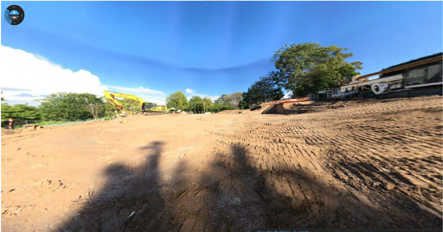
Photo 4 – The panoramas below show the site as at the 6 th of April with excavators performing excavation in the Southern corner of the site.
