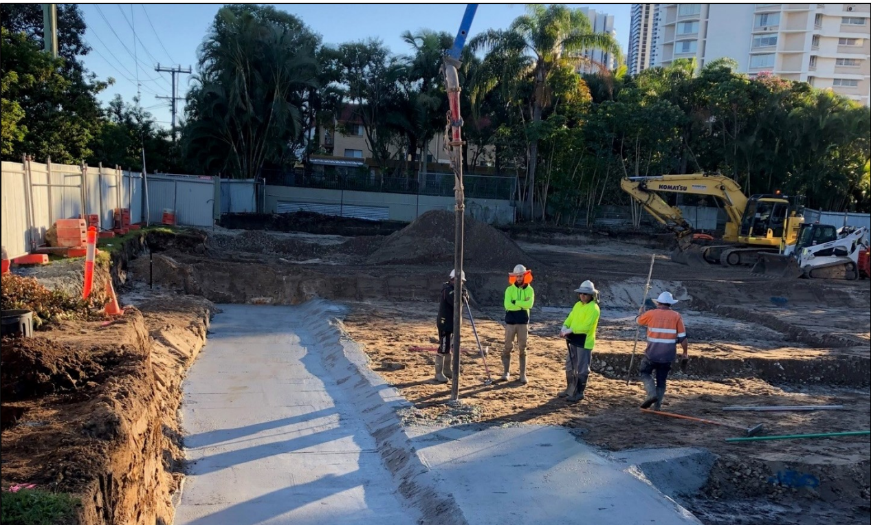
Peninsular Site: The blinding layer is poured over the sand base layer.
